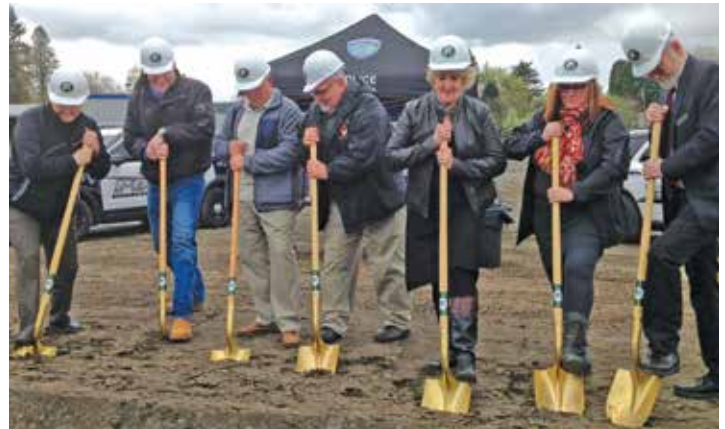
Gladstone Mayor Tammy Stempel and City Council members Matt Tracy, Randy Ripley, Neal Reisner, Linda Neace, Tracy Todd, and Thomas Mersereau (left to right) donned hardhats and took up golden shovels to break ground on the new Gladstone Police Station and City Hall.
