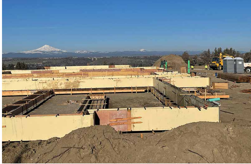
The Yarrow Apartments in Madras, the first of three phases of development to construct 148 units of market rate apartments. They are the first market rate apartments to be constructed in over 10 years. Photo courtesy of city of Madras.
