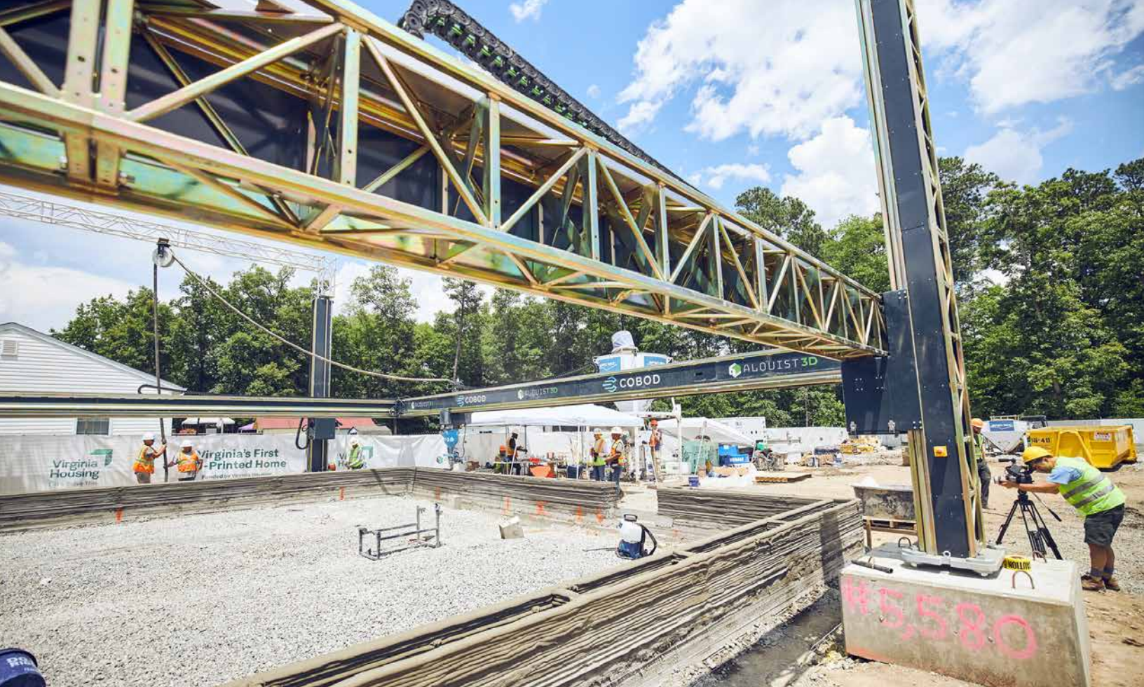
The first 3D printed homes in Oregon will be The Ridge in John Day, a master-planned development overlooking the John Day River. The Ridge will provide veteran's preference housing at a target rental rate of $850 per month. Photo courtesy of Town of Lakeview.
